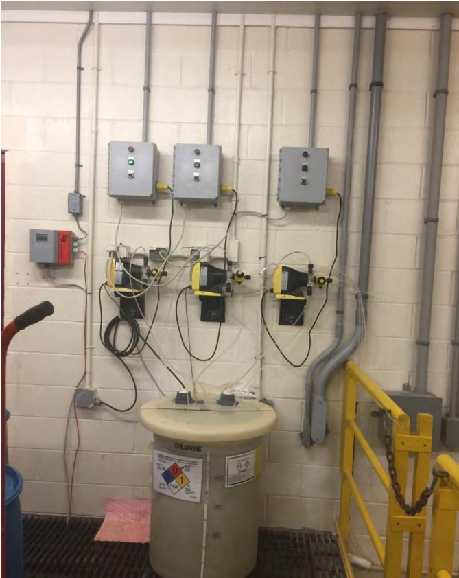
Water System Components: Pumps and Electrical
