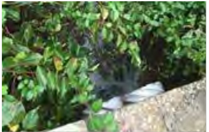
Storm Water Drainage
