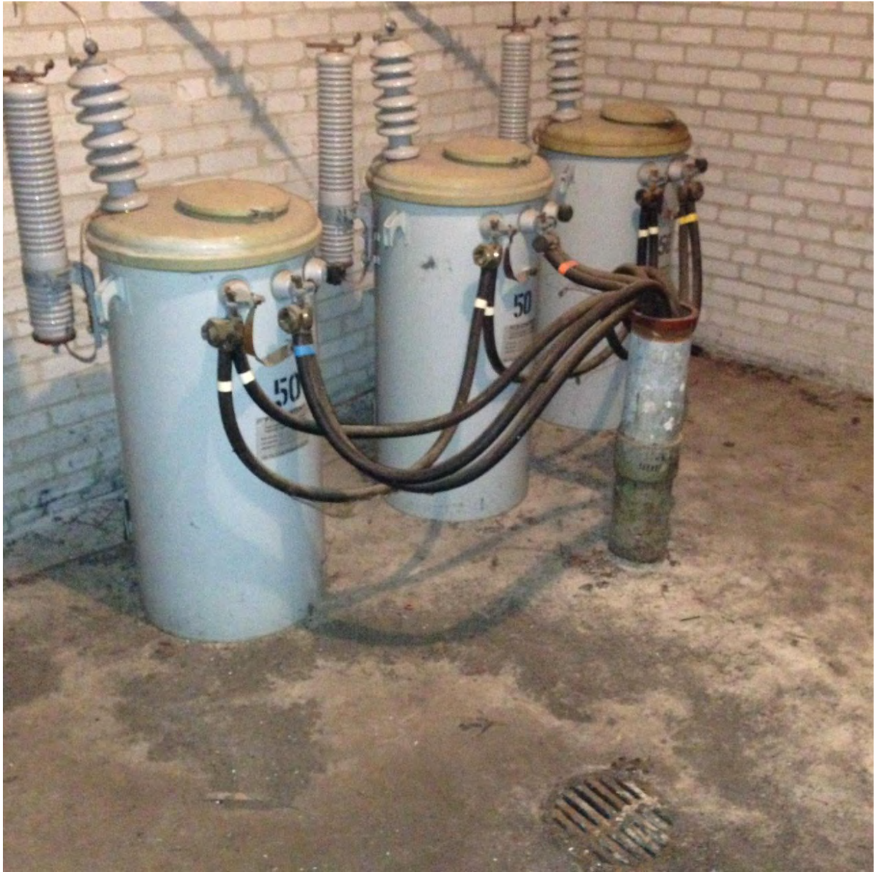
Typical Underground Transformer Vault
