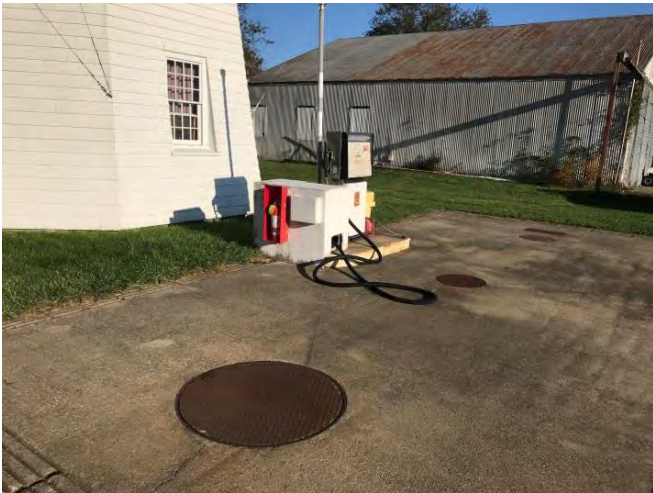
Cape Cod Air Field Fuel Tank Pump
