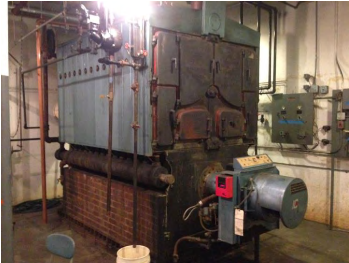
Cotuit Elementary School Boiler
