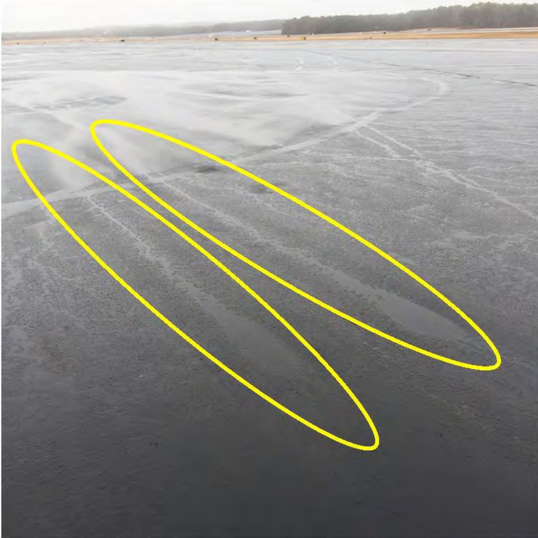
Pavement depressions due to heavy aircrafts
