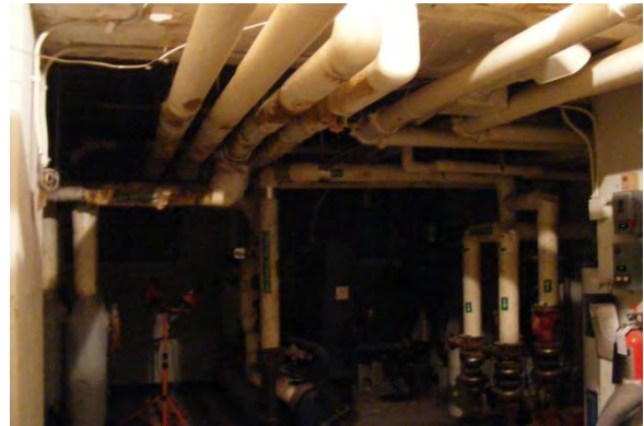
Mechanical Induct system
