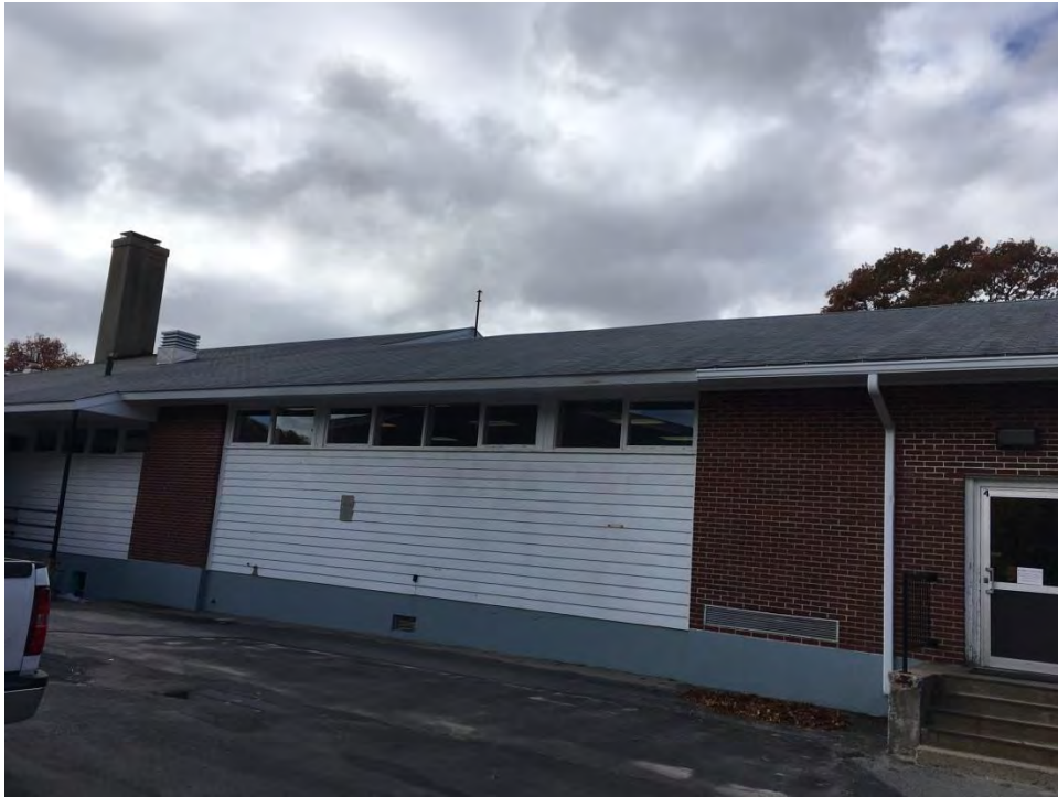
Centerville Elementary School Needs Roof Replacement
