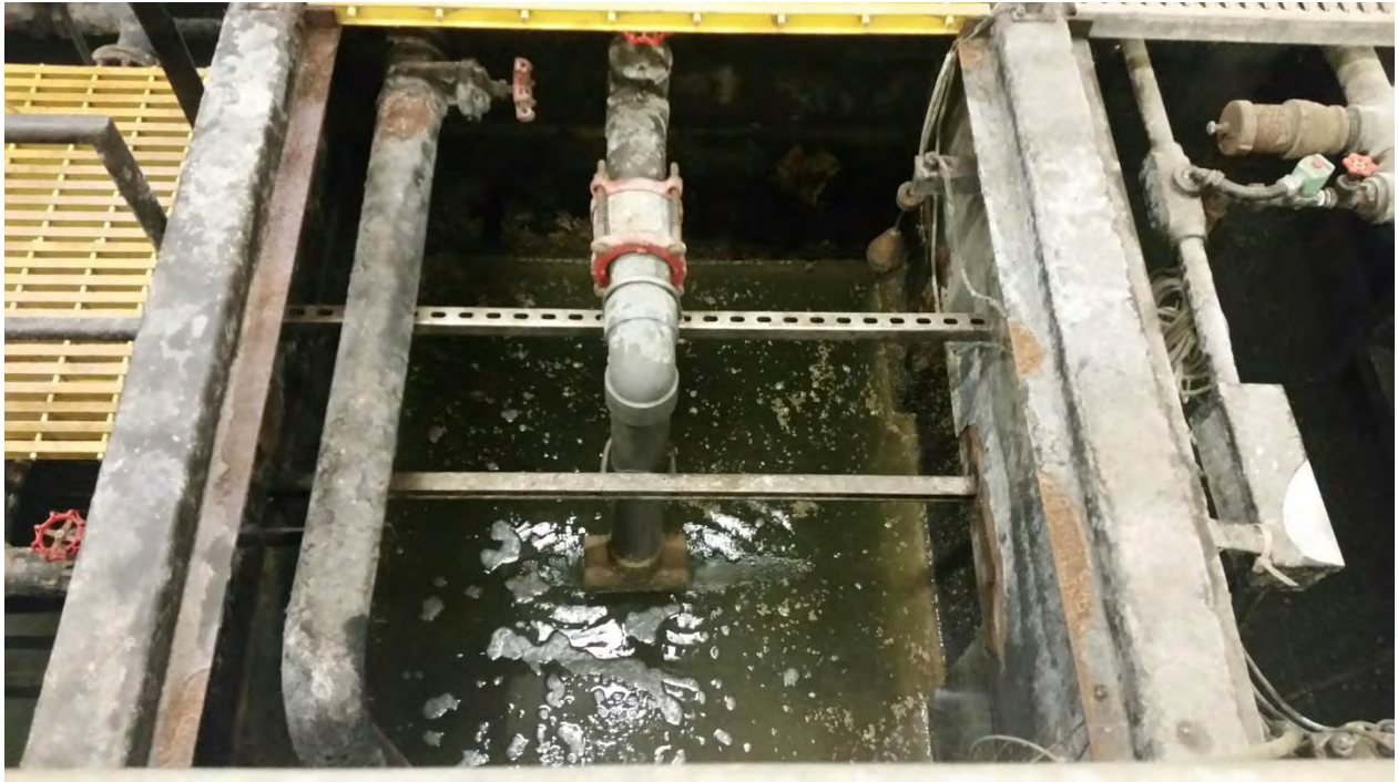
Denitrification Sand Filter
