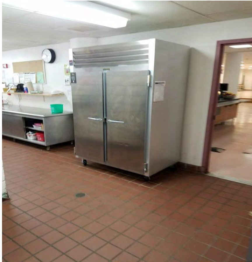
Barnstable Intermediate School Reach-In Freezer
