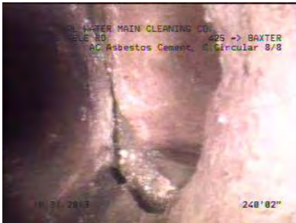
Barnstable Road Deteriorating Pipe
