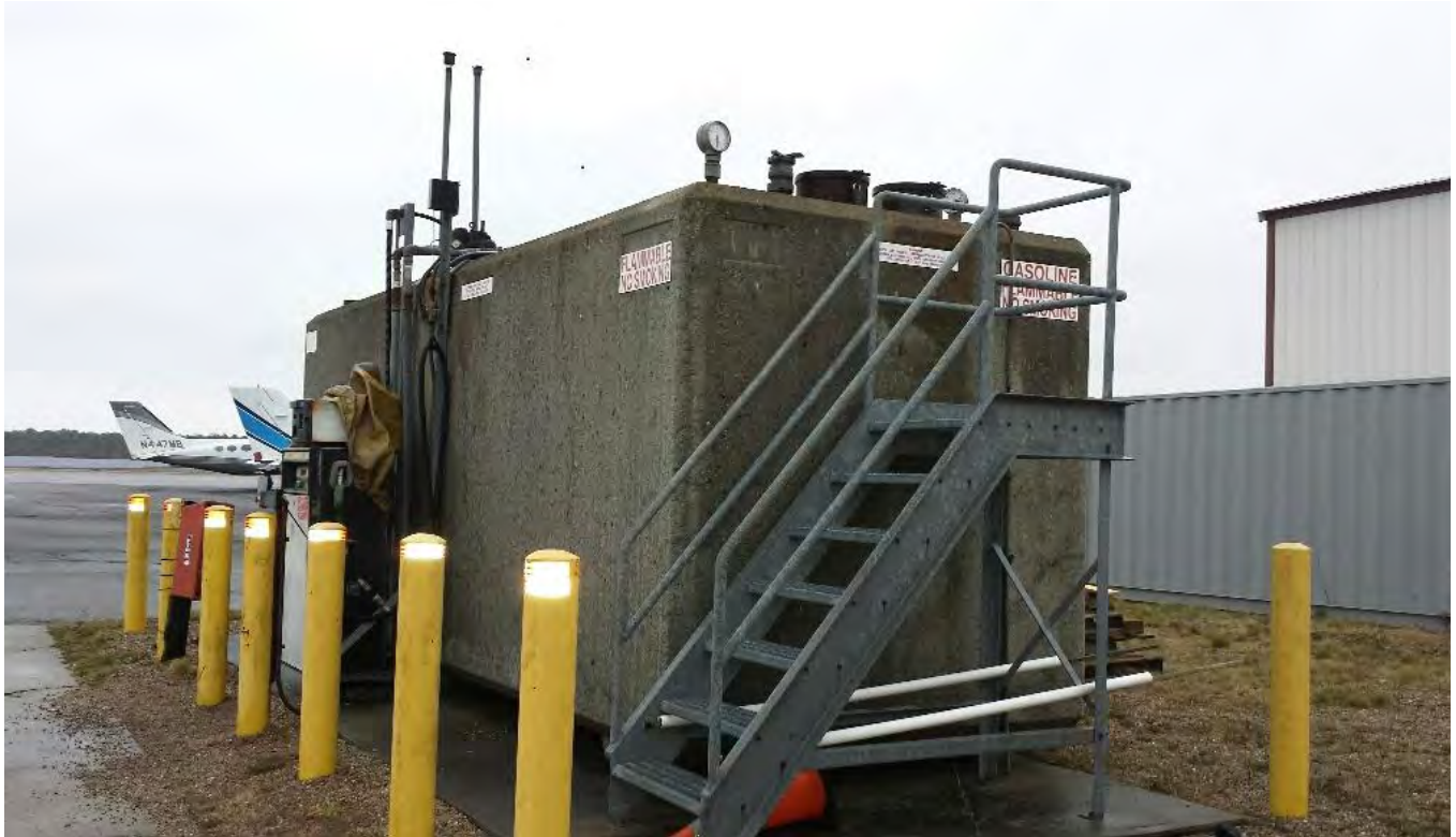
Mo-Gas and Diesel Fuel Con-Vault
