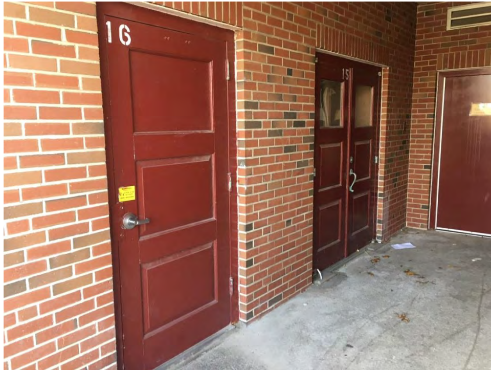
Hyannis West Door Needing Replacement
