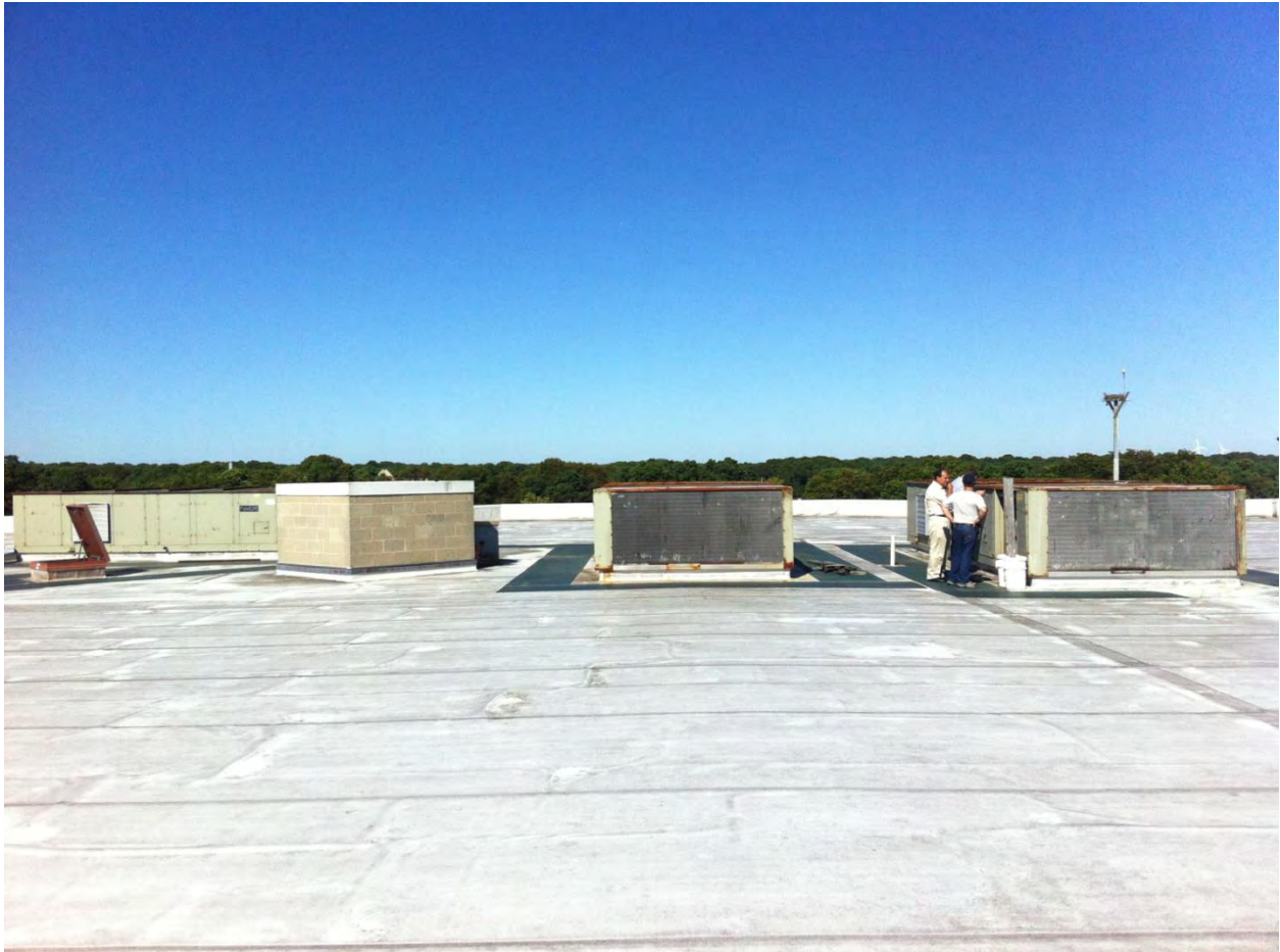
Roof Top Unit Ventilators (RTU)
