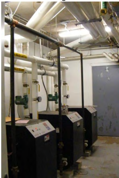
Mechanical Controls to Cooling System
