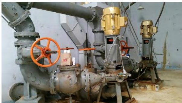
Freezer Road Pumps
